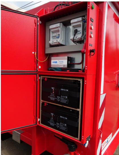
Electric switch cabinet
