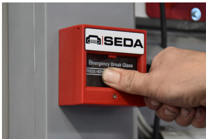
Manual activation of the fire alarm system
